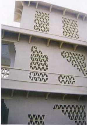
The architect sees the triangles in the jaali as a translation of her experience with the black bucks — the patterns formed in the landscape by the animals and their antlers as well as the patterns inherent in local crafts that come from black buck folklore
