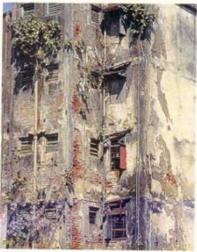
An example of not so old public housing by the Housing Board in Bombay. The design of such buildings reflects a singular concern for meeting cost ceilings at the initial stage beyond which it is a case of wasted resources. A poor and unresponsive agency fails in maintenance and repair of such indifferent buildings, as also do the users.
